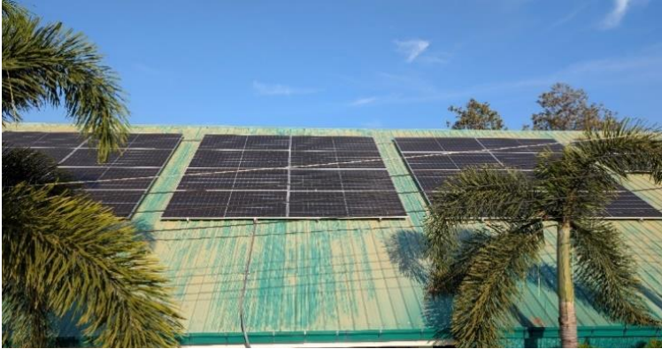
Solar panels installed on Life Centre
